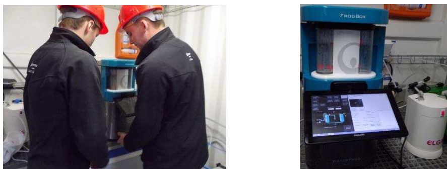
Figure 2. Installation of Frogbox for the assessment of the Actiflo® Carb effluent quality.
